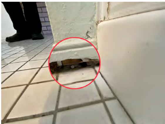
Fungal decay to timber skirting at shower
