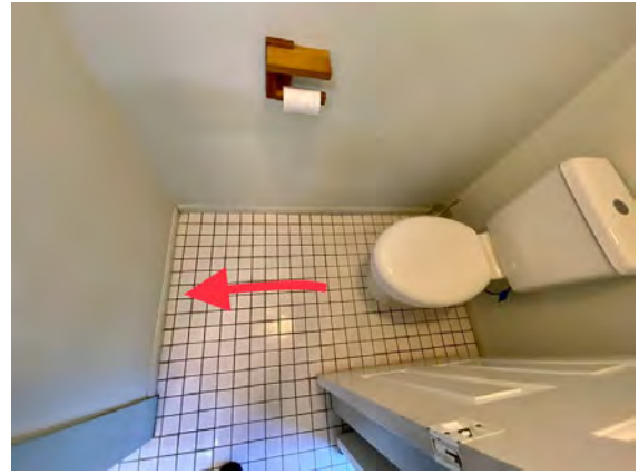
High moisture reading to toilet wall (adjacent to shower)
