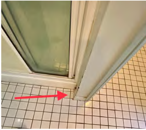
Apparent leak from shower tray when in use
