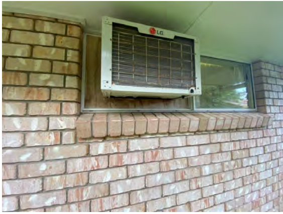
Air con overflow not connected to drain
