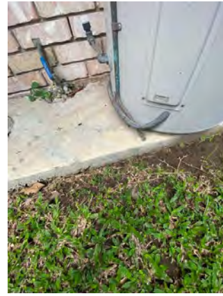
Hot water system overflow not connected to drain
