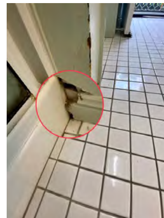
Fungal decay to timber skirting at shower
