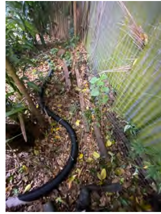
Timber on ground, mulched gardens, timber fencing in contact with soil
