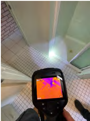
Apparent leak from shower tray when in use
