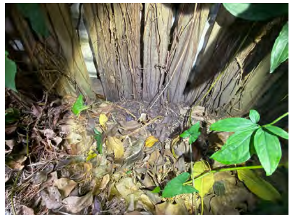
Mulched areas, timber fencing in contact with soil
