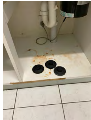
Some apparent water damage under kitchen sink- appears previous
