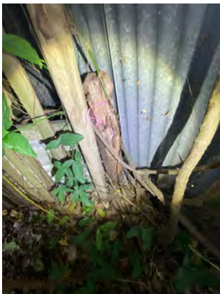
Termite damage to timber fence post - back yard
