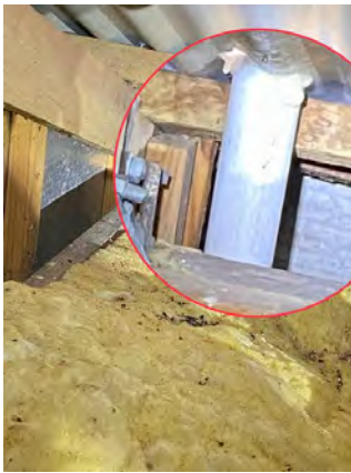
Some water stains to timber around vent pipe (bedroom 1) appears previous
