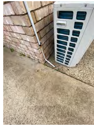
Air con overflow not connected to drain
