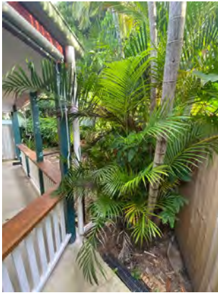
Trees/Vegetation in contact with structure, mulched gardens present
